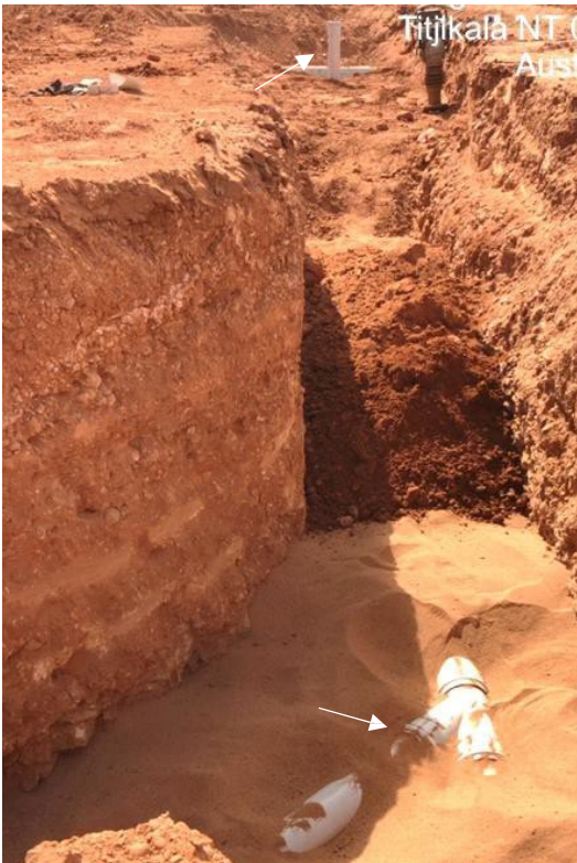
Above: Riser at main (top of image), junction for dual lot servicing (if relevant) and both risers visible.
