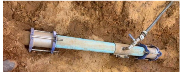
Above: AC replacement for new water service (no cutting of AC permitted).
