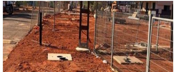
Above: Showing both IO covers associated with the installation for the specific lot.
