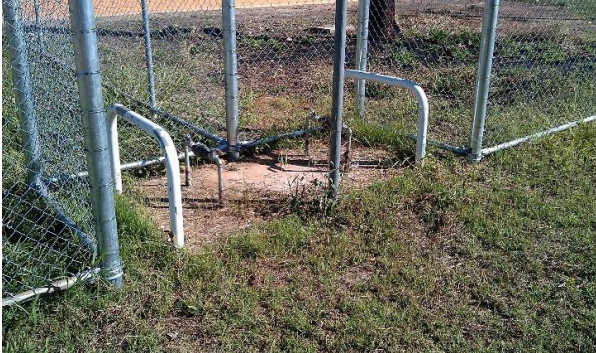
Above: Water meters or fence incorrectly installed.
