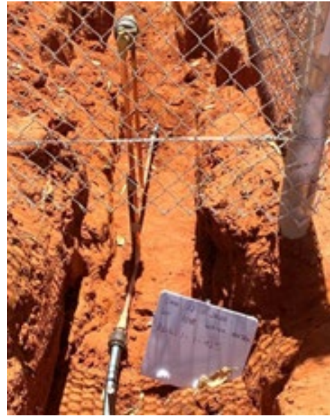
Above: Connection between underground pipework and above ground copper riser.
