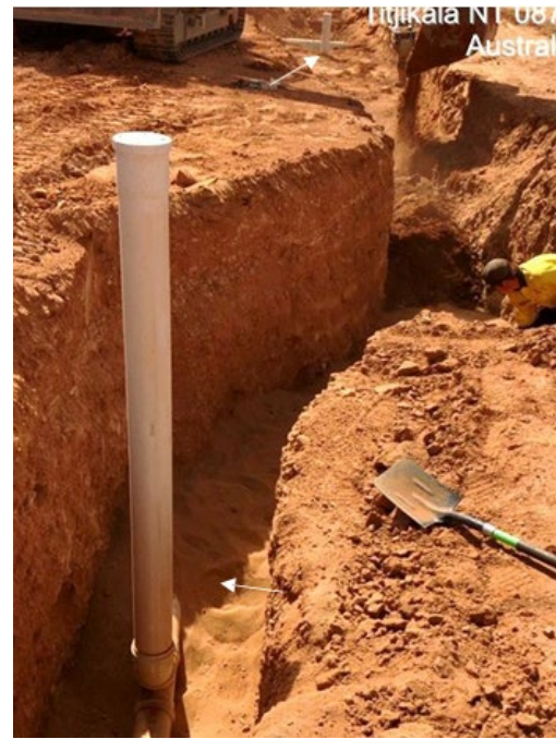
Above: Riser at main (top of image), junction for dual lot servicing (if relevant) and both risers visible.
