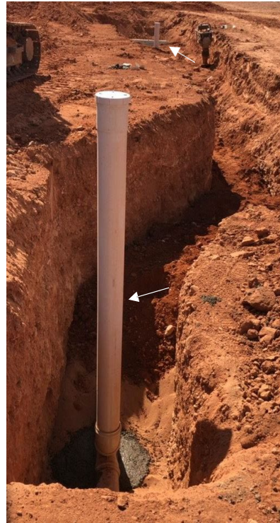
Above: Riser at main in distance (top of image), junction for dual lot servicing (if relevant) and both risers clearly in one image.
