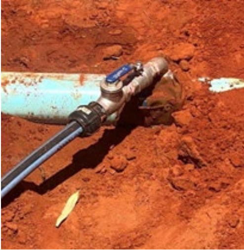
Above: Non-aggressive water installation (ROW1-1-425).
