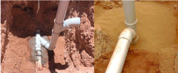
Above: Riser at main with thrust block in place and continuation of pipework from riser.
