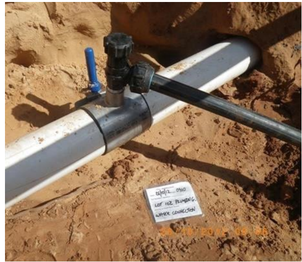
Above: Incorrect PE tapping to water main.
