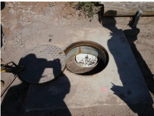
Above: Sewer MS IO lid incorrectly aligned.
