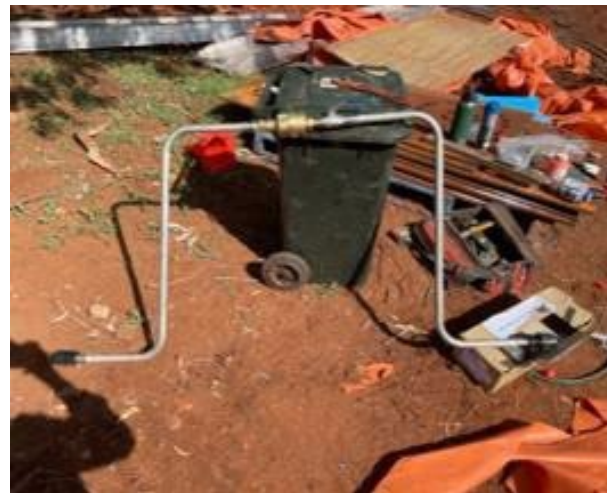
Above: Incorrect extended water assembly.
