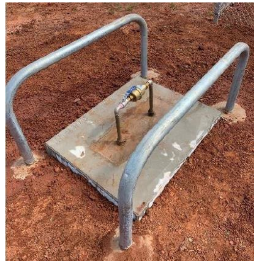
Above: Completed meter arrangement (ROW1-1-325).
