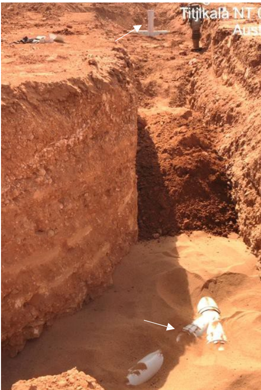
Above: Riser at main in distance, junction for dual lot servicing (if relevant) and both risers clearly in one image.
