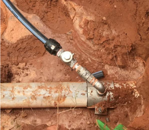
Above: Aggressive water installation (ROW1-1-325).
