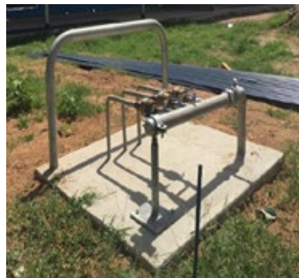
Above: ROW1-1-350 for triplex servicing (W1-1-18A)
