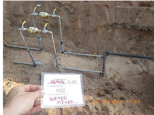
Above: Connection between the underground pipework and above ground stainless steel riser for Duplex (W1-1-25).
