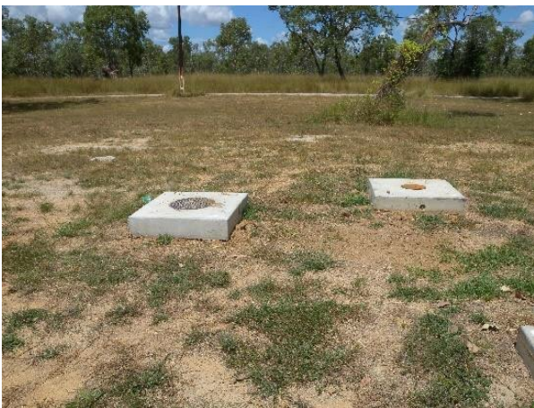
Above: Sewer IO's incorrectly installed.
