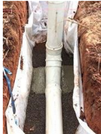
Above: Concrete thrust block at riser.
