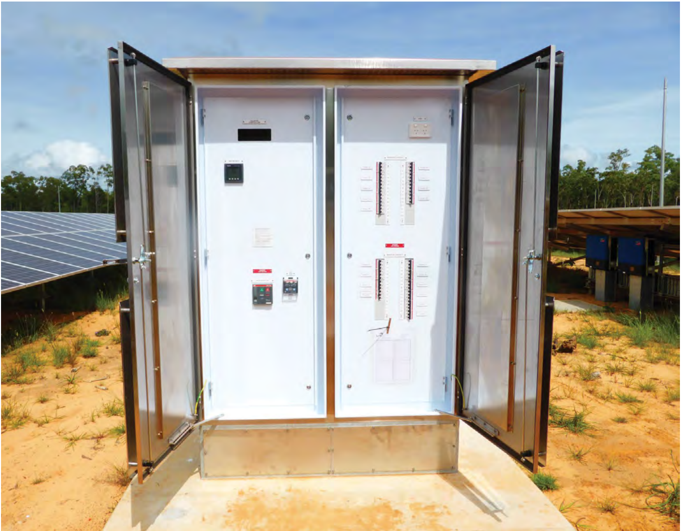
Figure 3 – PV LV Switchboard at Maningrida array #2
