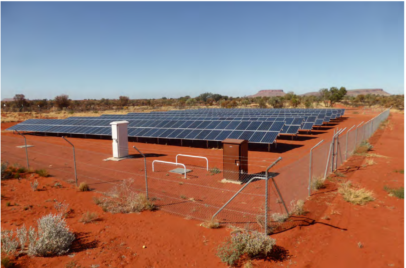
Figure 7 – The SETuP solar array at Mt Liebig
