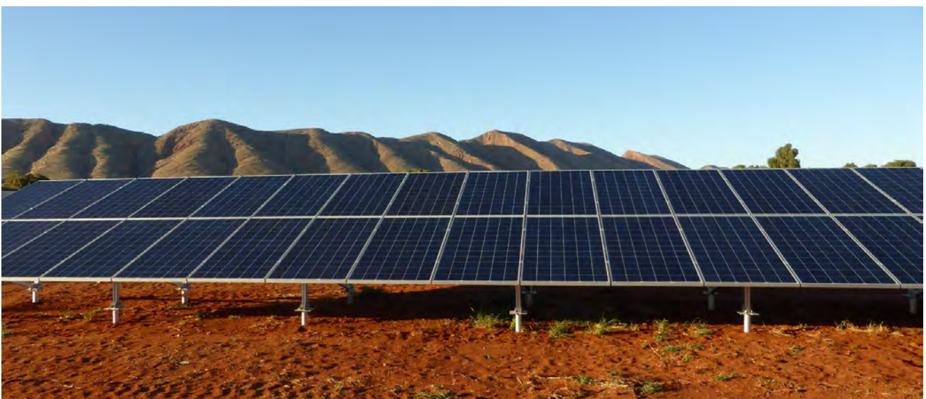
Figure 5 – The SETuP solar array at Kaltukatjara (Docke River)
