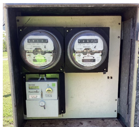
Figure 3.1: Example of three single phase meters
