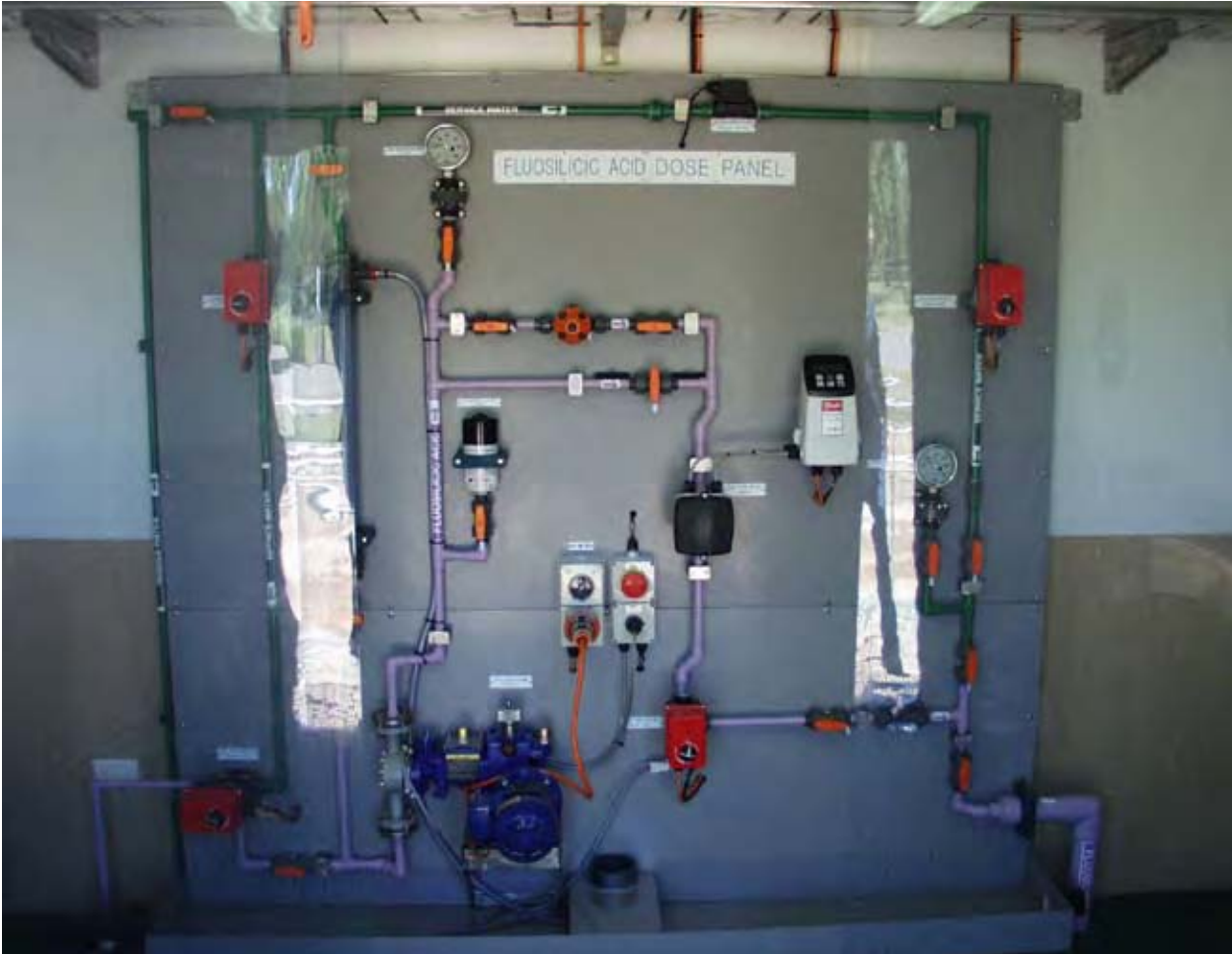
FLUORIDE DOSING AND MONITORING AT DARWIN RIVER DAM
