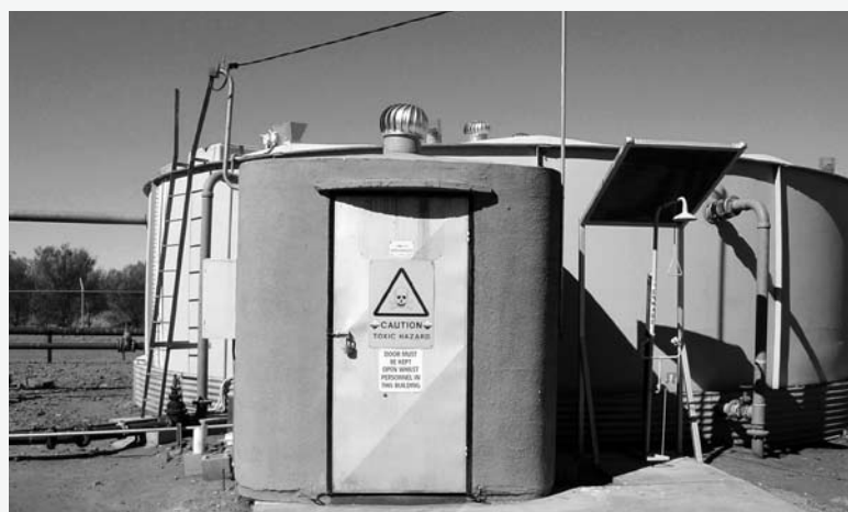
GASEOUS CHLORINE STORAGE FACILITY, KINGS CANYON.
