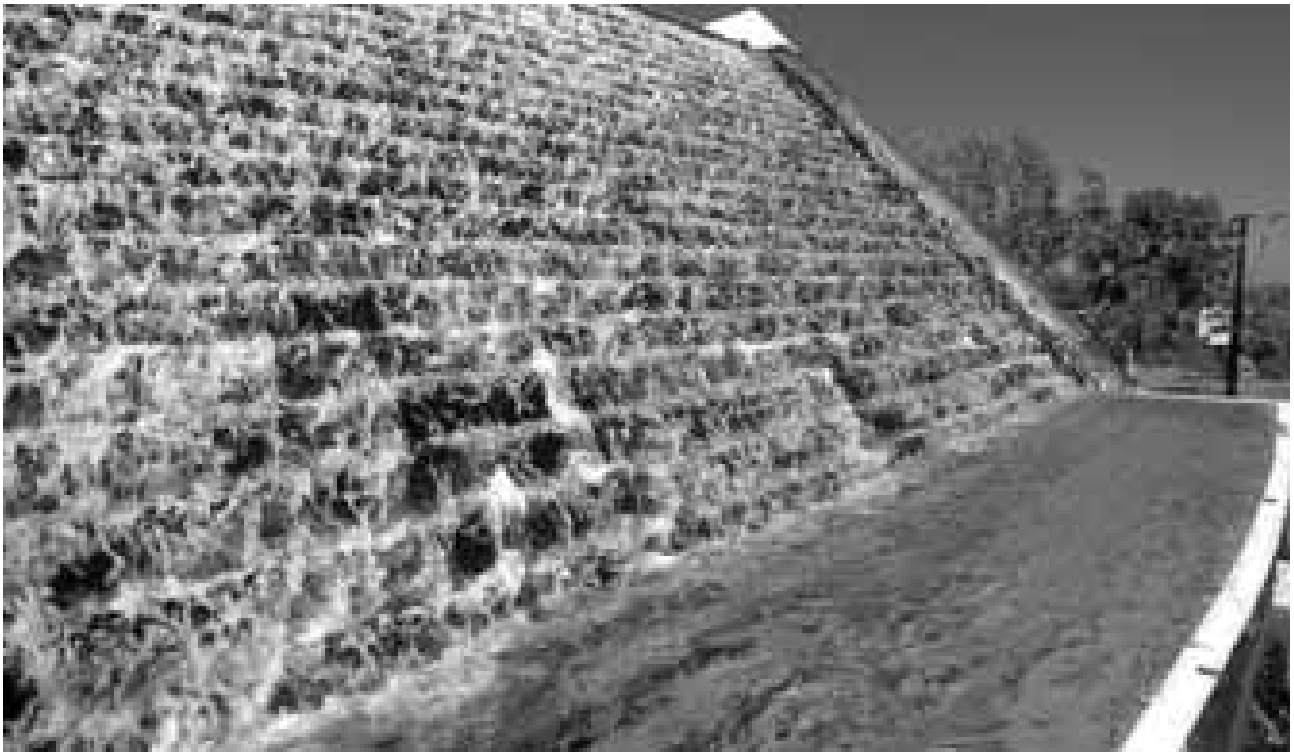
GROUND WATER AERATION AT THE KATHERINE WATER TREATMENT PLANT
