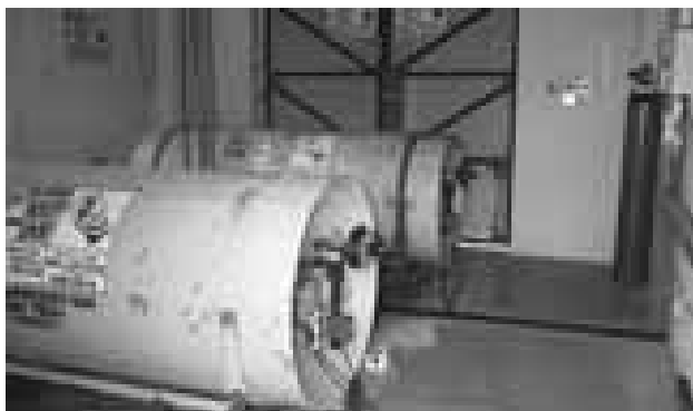
GASEOUS CHLORINE DRUM STORAGE
