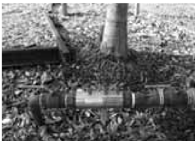
BACK-FLOW PREVENTION DEVICE ON WATER METER
