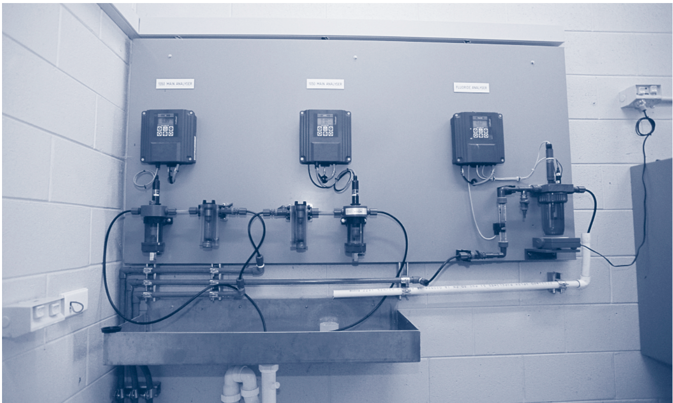
On-line Water Quality Analysis at Darwin River Dam.
