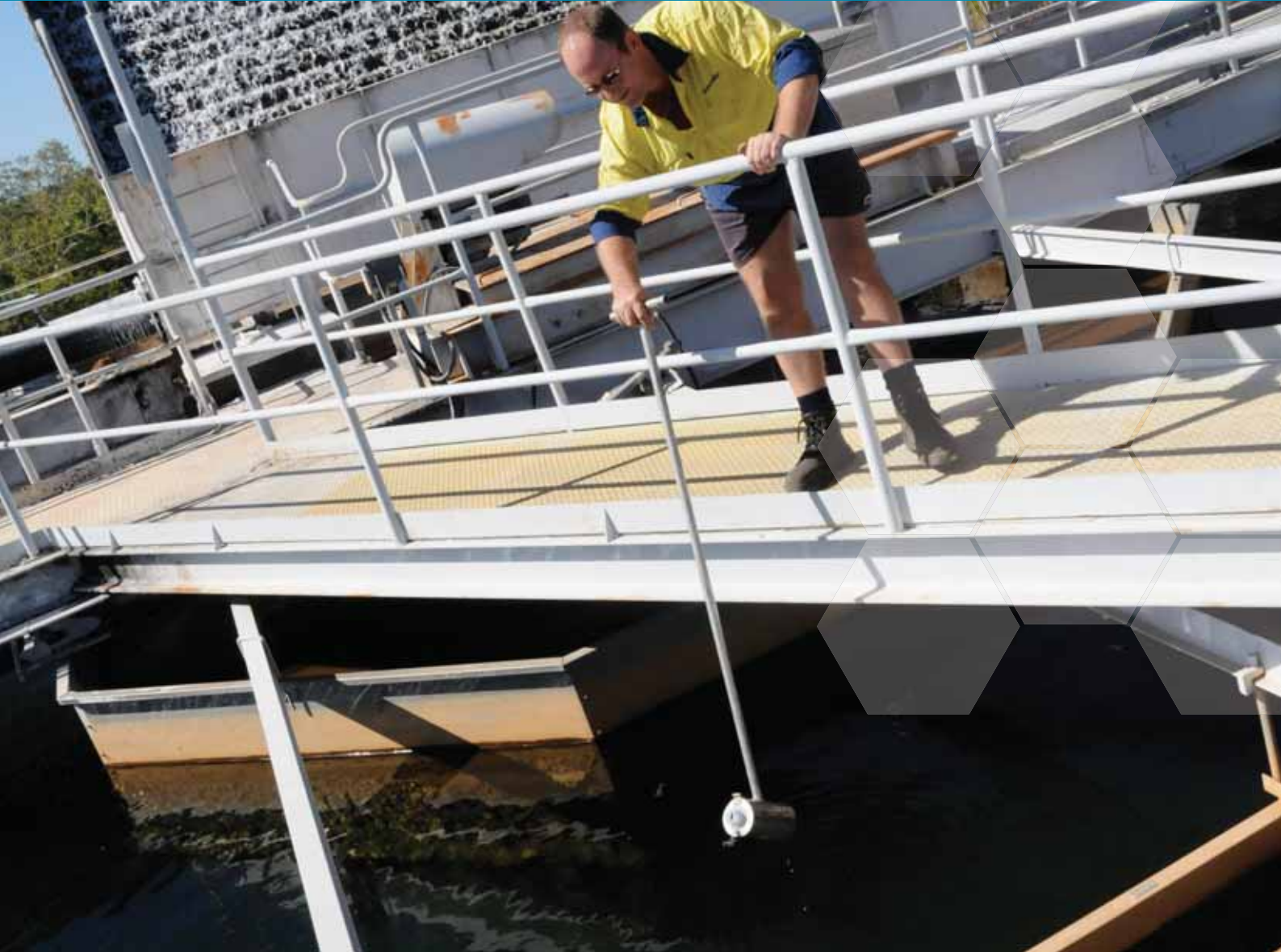
ABOVE ► JASON BIRD COLLECTING A WATER SAMPLE FROM THE CLARIFIER AT THE KATHERINE WATER TREATMENT PLANT
