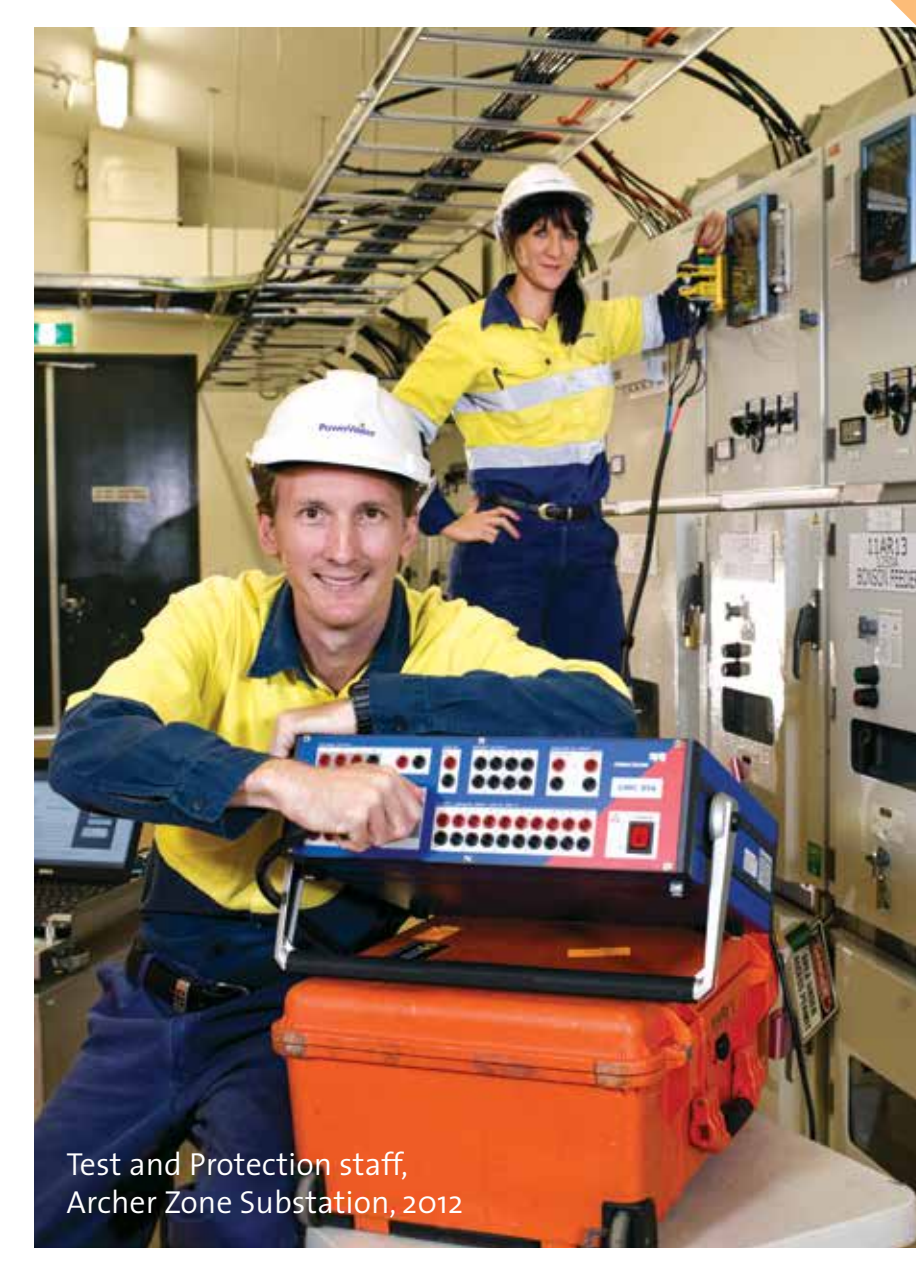
Test and Protection staff, Archer Zone Substation, 2012
