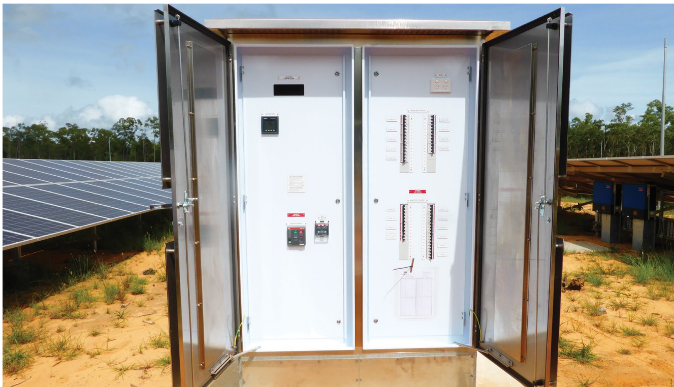
Figure 3 – PV LV Switchboard at Maningrida array #2
