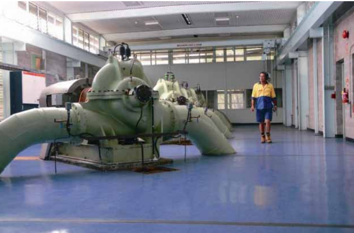
Darwin River Reservoir pump-station.
