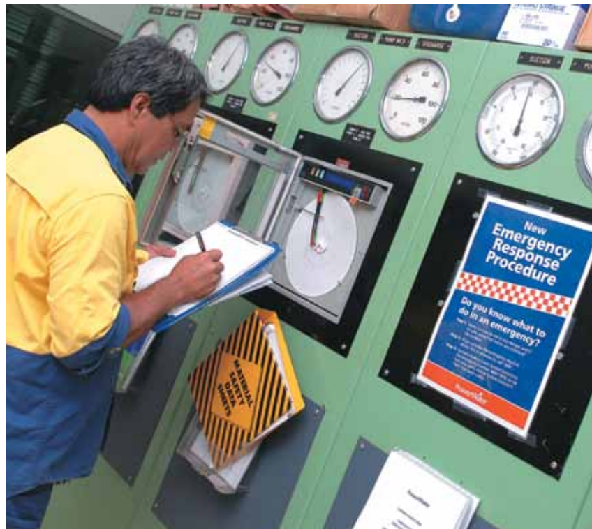
BELOW ► WATER FLOW RECORDING. DARWIN RIVER RESERVOIR PUMP STATION
