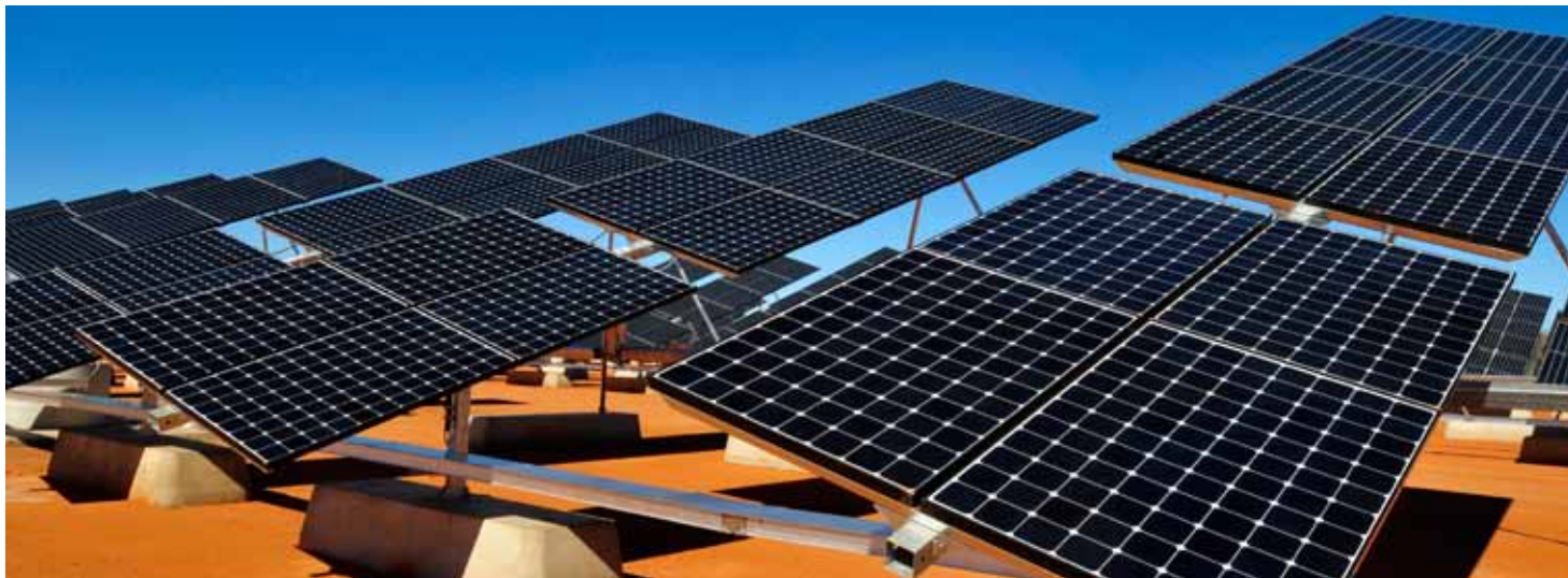
Flat-plate solar panels track the sun at Uterne in Alice Springs.
